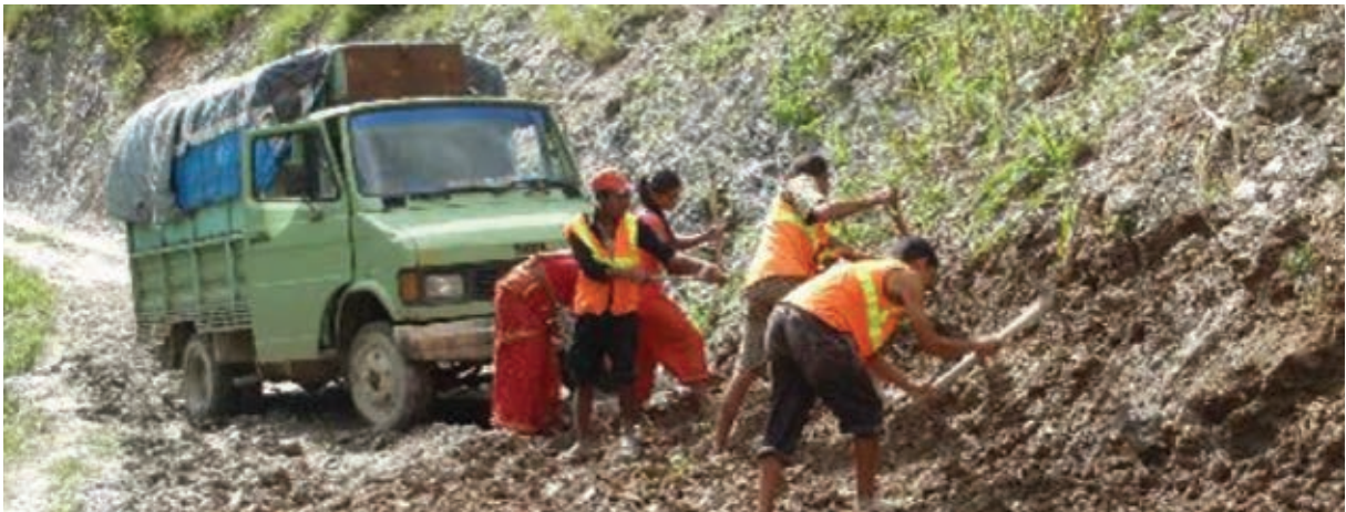
Emergency maintenance to allow traffic to pass critically problematic section of the road
