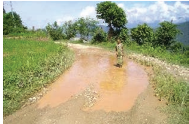
Water stagnation in pothole
