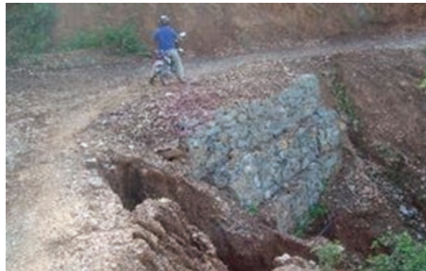
Gully formation in the road shoulder
