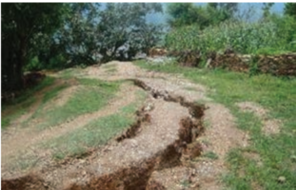
Erosion of the road surface
